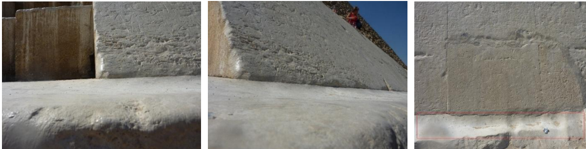
Figs. 9 and 10 Wear of the paving immediately outside the cladding blocks at point 3, in Fig. 11 highlighted in the red rectangle.
