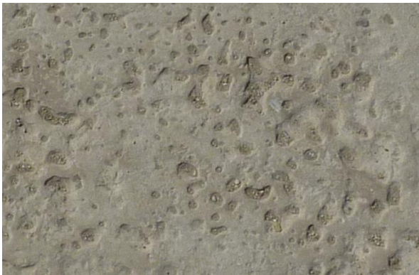
Fig. 2 Pitting erosion on limestone rock.
