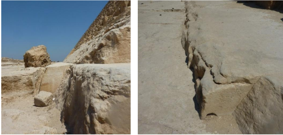
Fig. 18 Wear or erosion of the paving immediately outside the cladding blocks at point 10, and, in Fig. 19, at point 11.
