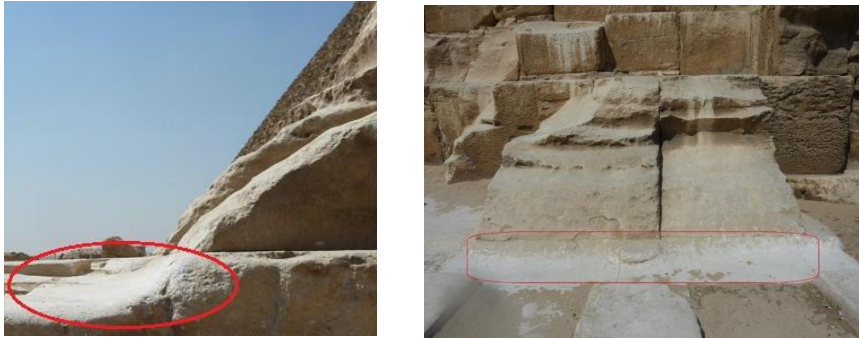
Fig. 12 Wear on the paving immediately outside the paving blocks at point 6, highlighted in the red oval, and in Fig. 13 in the red rectangle.
