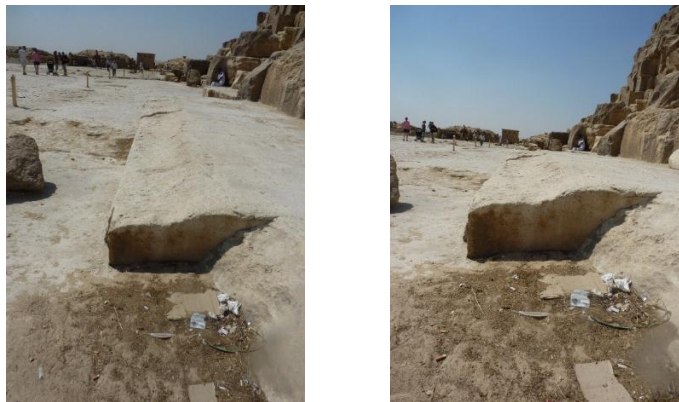
Figs. 14 and 15 Wear or erosion of the paving immediately outside the cladding blocks at point 7.
